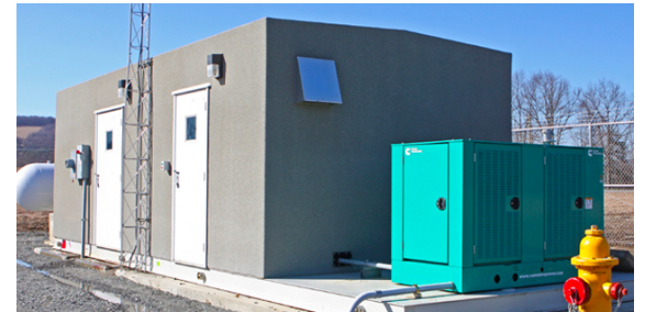
Savona Pump Station
