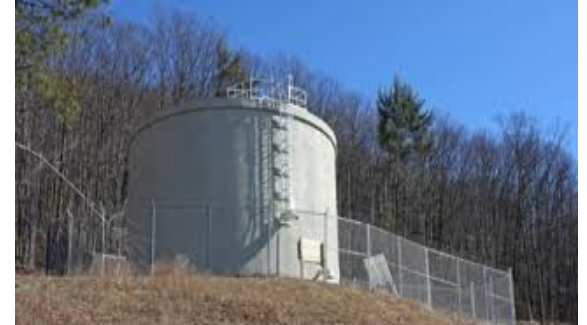
Water storage vessel in Savona
